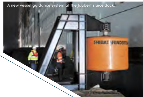
A new vessel guidance system at the Joubert sluice dock.
